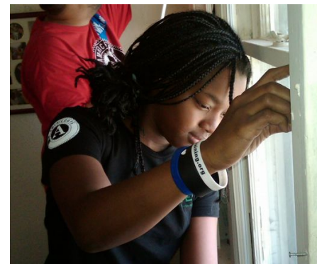
A YES crew member installs a window kit to keep a family warm.
